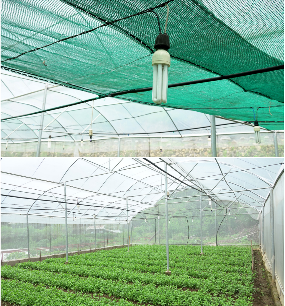
Fig. 14. Installation of 40-watt light bulbs at a height of 5.0 ft. above ground at distance of 2 meters.
